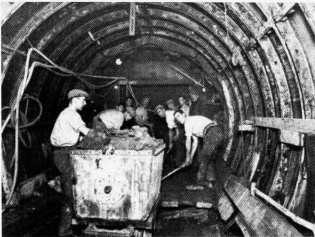
Underground tunnelling work in progress near Finsbury Park on the Southgate extension of the Piccadilly line. Several tunnel miners are at work at the tunnel face within a Greathead shield
